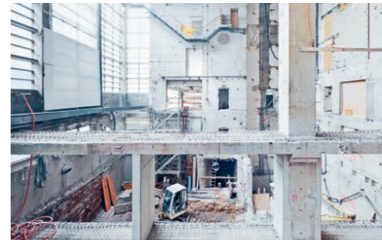
The Machinery Laboratory/District Heating Plant (ML/FHK) belonging to ETH Zurich at Zurich Zentrum – a refurbishment performed under strict heritage conservation regulations.
